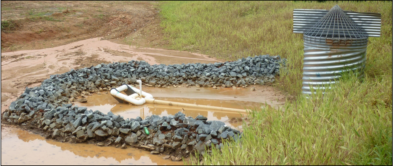
Photo: Horseshoe Rock Berm Around Principle Spillway with Skimmer
