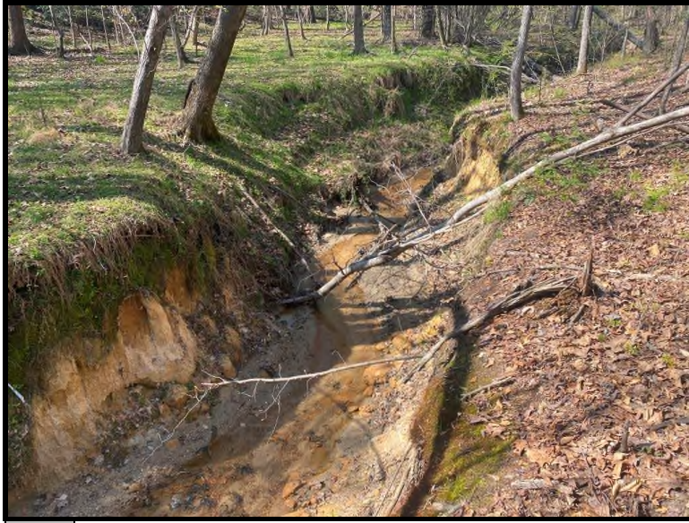
21 Intermittent tributary located on the eastern portion of the site. Severely eroded banks.
