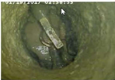
Lead Service Line
