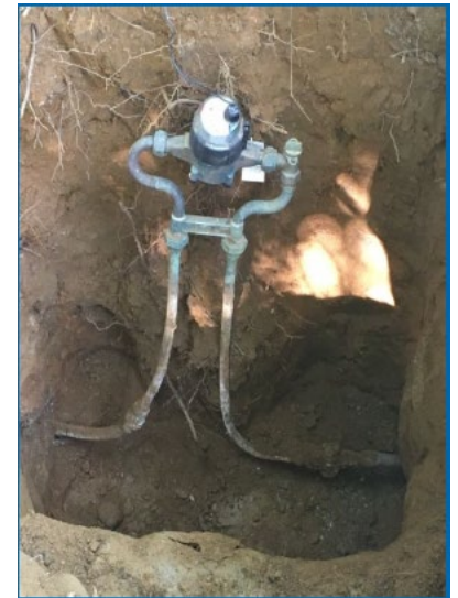
Example of Meter Pit Source: LSLR Collaborative 2018
