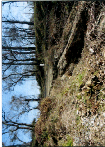
View of the end of Senate Street Extension from alluvial fan (Note eroded area that will require reconstruction)
